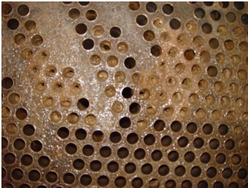
Scaling on condenser tubes before cleaning
