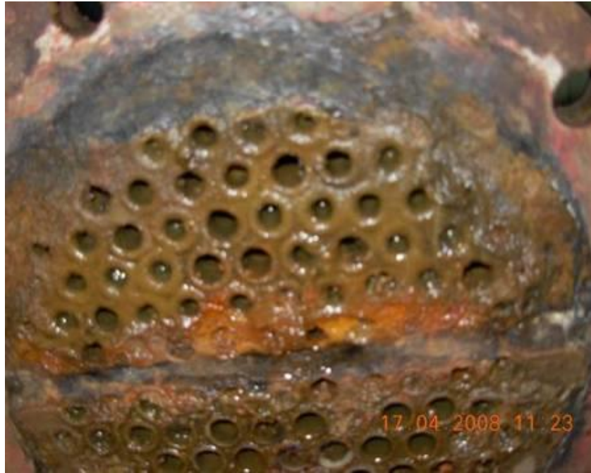
Scaling on condenser tubes before cleaning
