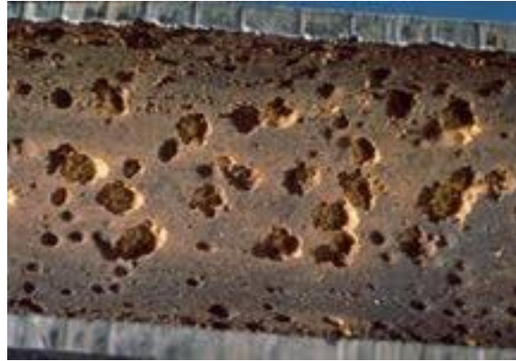
Pitting Corrosion Under Colloidal Iron Stagnation
