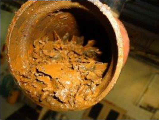
Stagnation of Colloidal Iron in Lines
